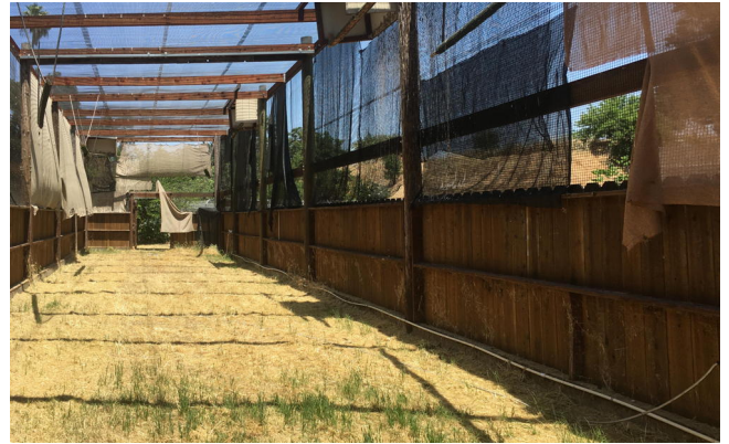
The eagle aviary before repairs. Although the basic structure is quite sound, the netting made it look as if it was about to fall down.
